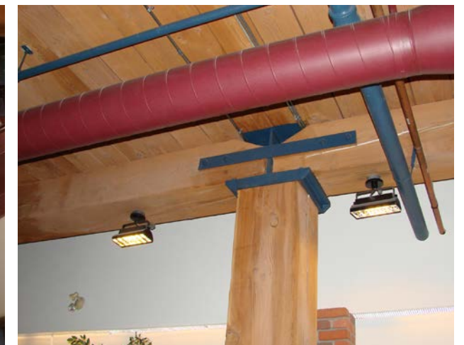
Figure 3.12 Structural connection with column cap at the Leckie Building Photo courtesy of FPIinnovations
