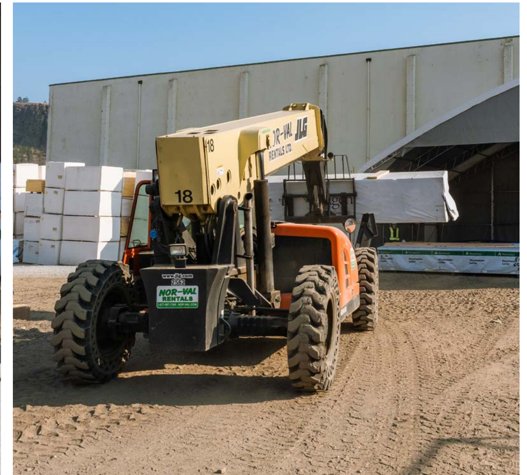
Below Unloading NLT panels Photo credit Bryce Byrnes Photo courtesy of NaturallyWood
