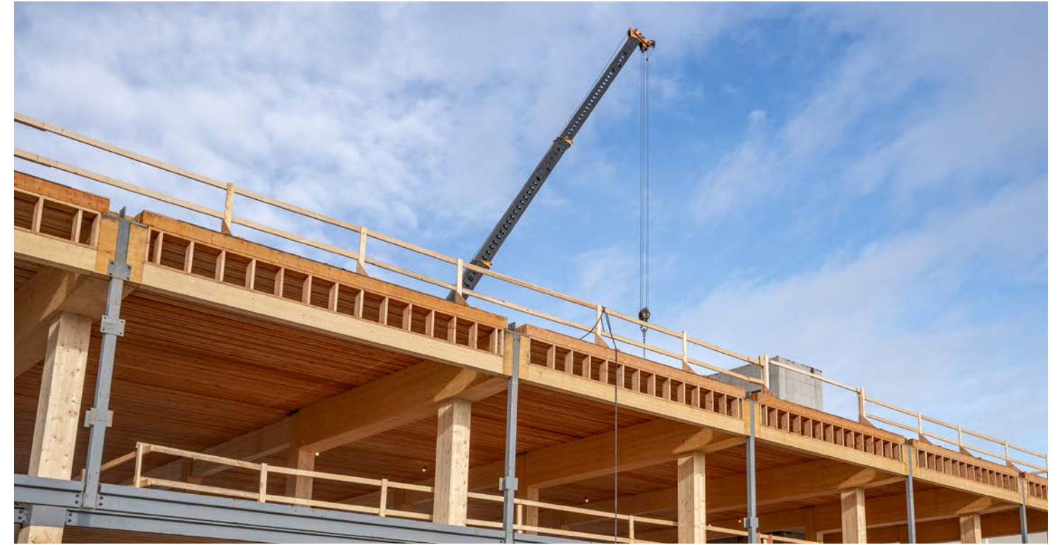
Above The Exchange, Kelowna, BC, during construction Photo credit Jason Harding Photo courtesy of NaturallyWood
