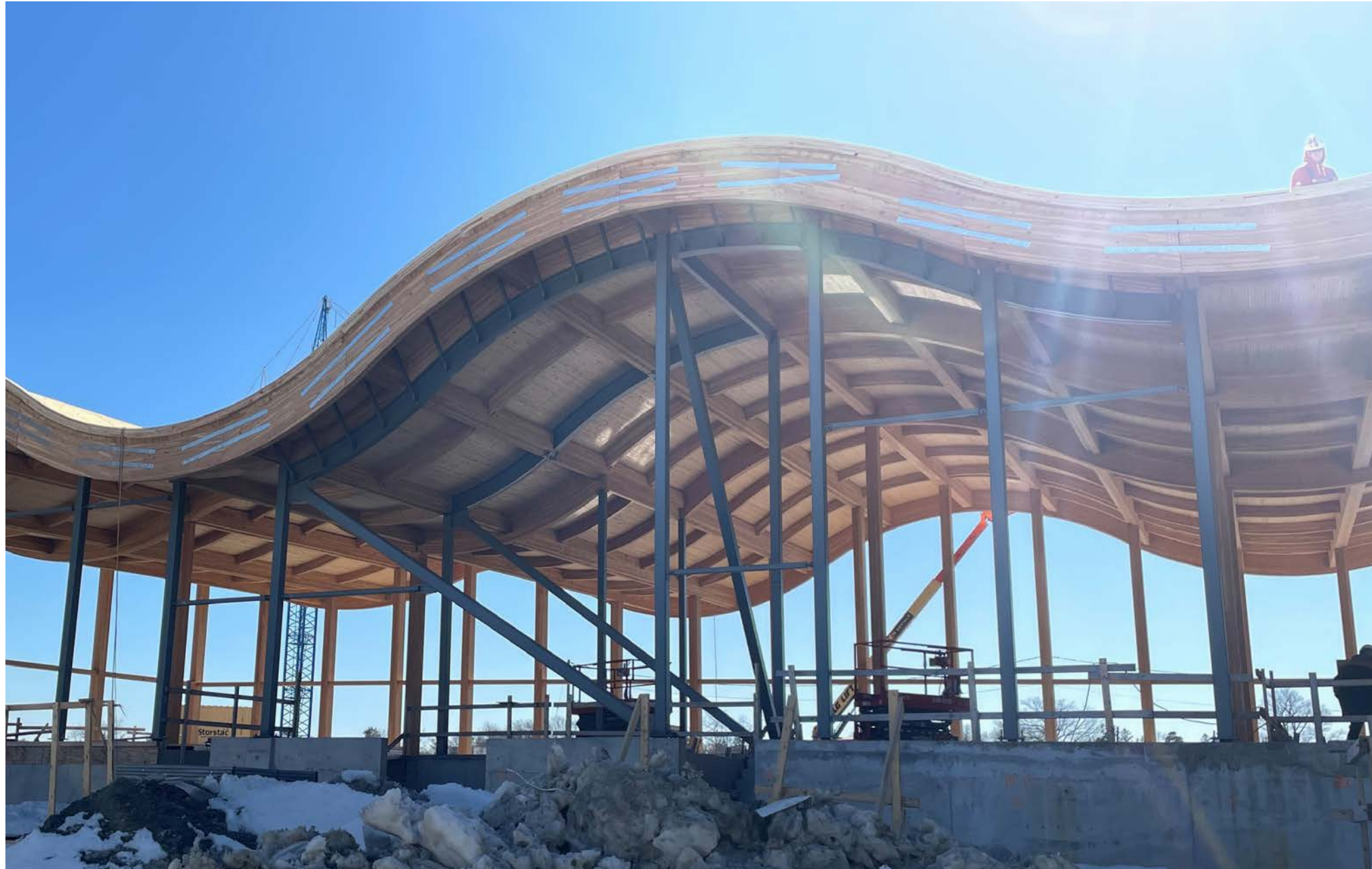
Above Brightwater C4 Building, Port Credit, ON, during construction Architecture by Diamond Schmitt Photo courtesy of Silvaspan
