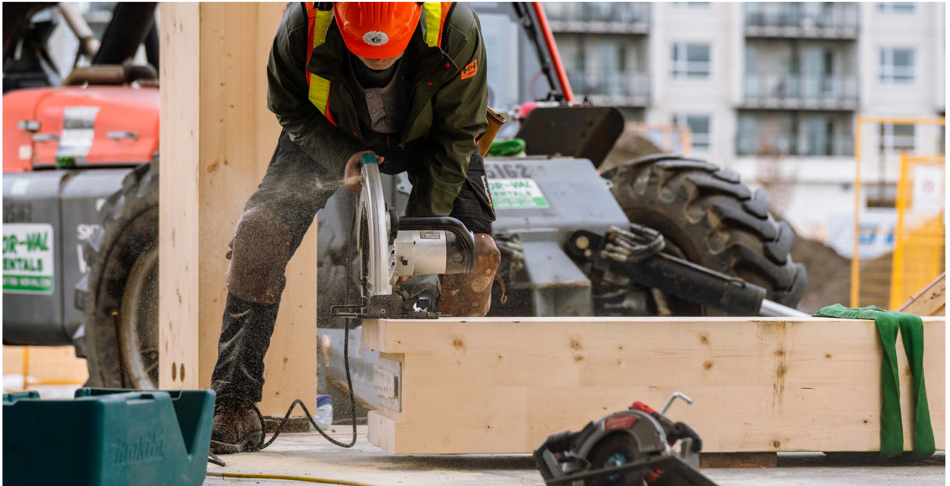
Above Cutting on-site, The Exchange, Kelowna, BC Photo credit Jason Harding Photo courtesy of NaturallyWood
