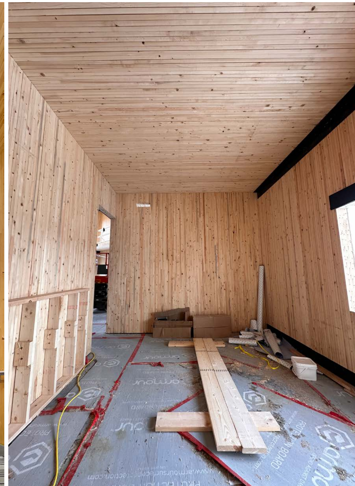
Below NLT walls under construction at 51 Kingston, Goderich, ON Photo courtesy of Silvaspan
