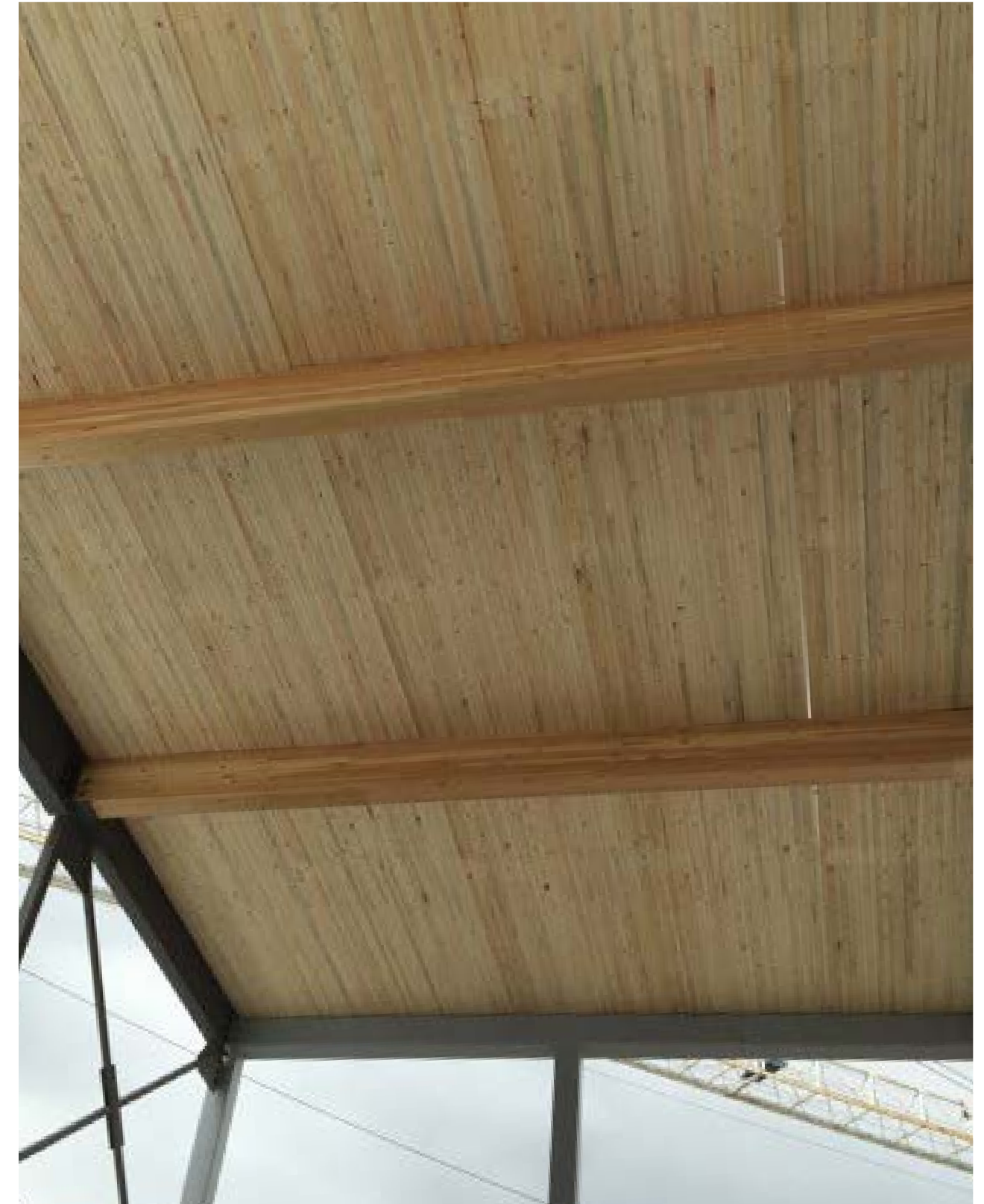
Figure 8.5 NLT install of prefabricated pre-sheathed panels Photo courtesy of Seagate Structures Ltd.
