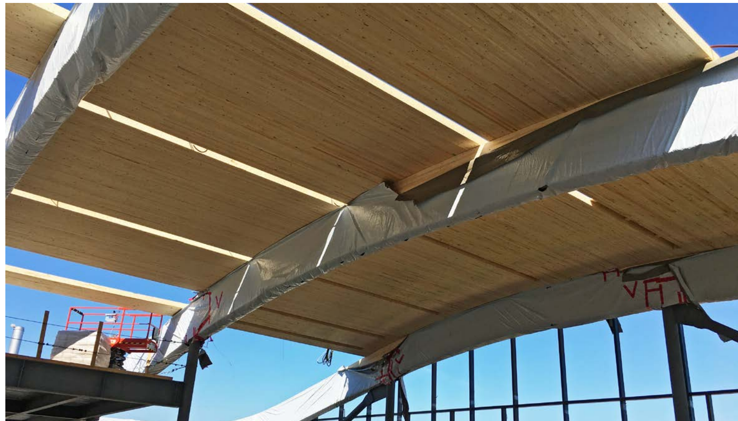
Below Algonquin College DARE District, Ottawa, ON, during construction Architecture by Diamond Schmitt Photo courtesy of Diamond Schmitt
