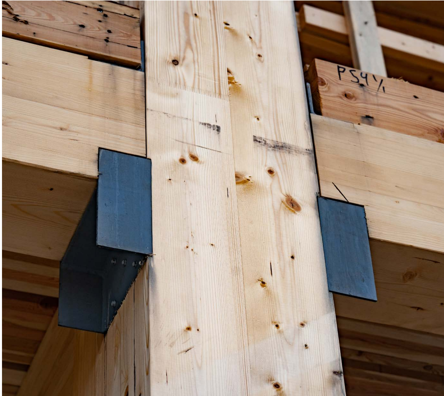
Above The Exchange, Kelowna, BC, during construction Photo credit Jason Harding Photo courtesy of NaturallyWood
