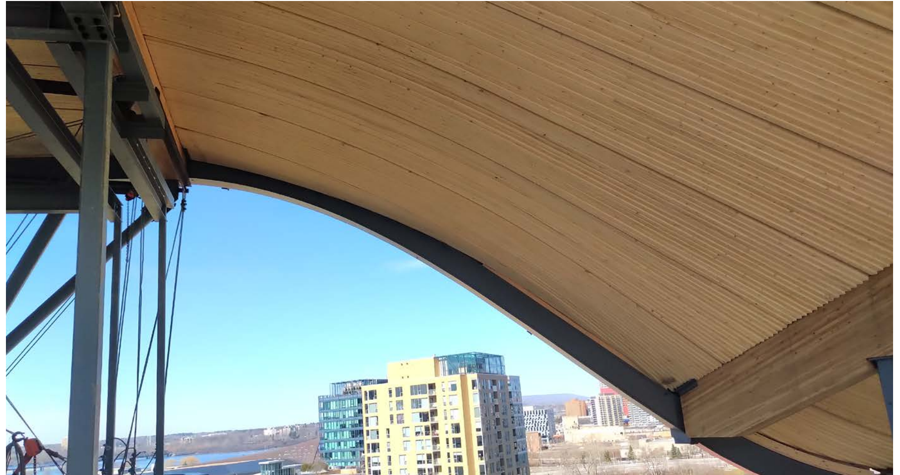
Figure 2.6b NLT with curved laminations, Ādisōke Public Library, Ottawa, ON Architecture by Diamond Schmitt Photo courtesy of Fast + Epp
