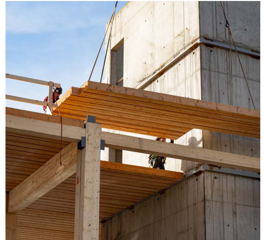
Above The Exchange, Kelowna, BC, during construction Photo credit Jason Harding Photo courtesy of NaturallyWood
