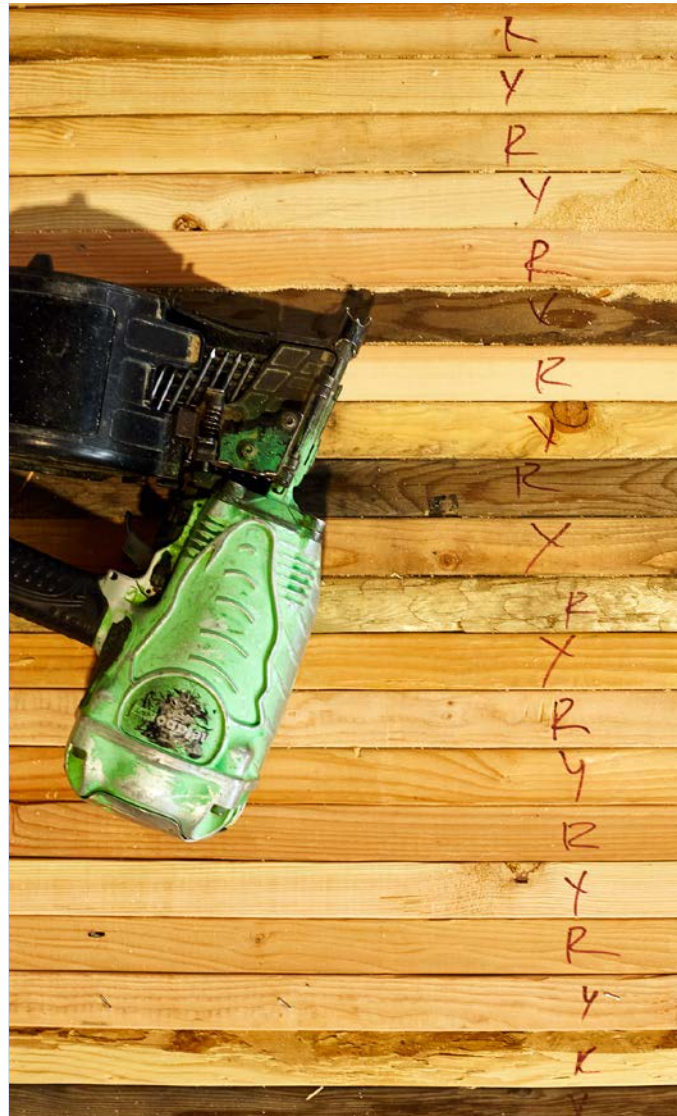
Above Testing nail order on NLT mock-up, The Exchange, Kelowna, BC Photo credit Wade Comer Photography Photo courtesy of NaturallyWood
