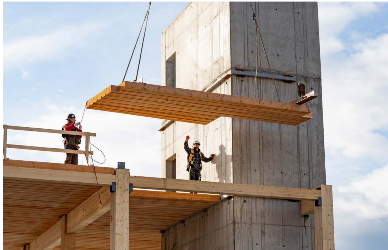
Below The Exchange, Kelowna, BC, during construction Photo credit Jason Harding Photo courtesy of NaturallyWood
